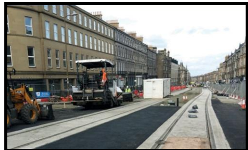
Trams are the most energy-efficient zero emission city transport. The photo above shows track laying on Leith Walk on the Edinburgh Tram extension to Newhaven.
